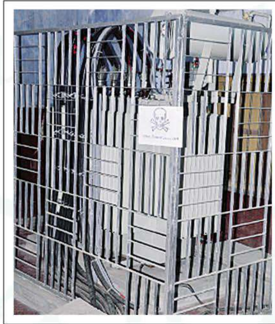
Newly built 11/0.415 kV, 1000 kVA electric Sub-Station at Mirzapur Complex.
